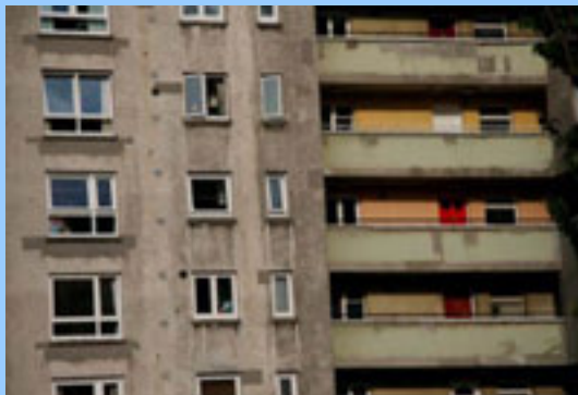
High rise blocks in poor condition
